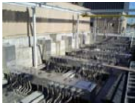
Commissioning DSRSD CA
